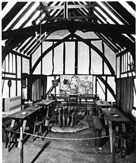
The Solar in 13th Century Southchurch Hall is a popular stop for visitors and residents alike.
